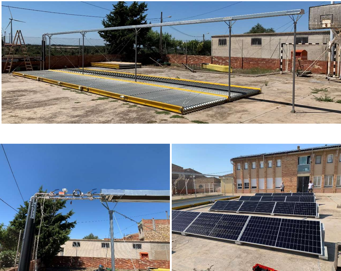
Figure 10. Outdoor system components in Almatret: solar thermal (top picture) and PV collectors (down-right), and details on hydraulic connection with the solar thermal collectors (down-left)
