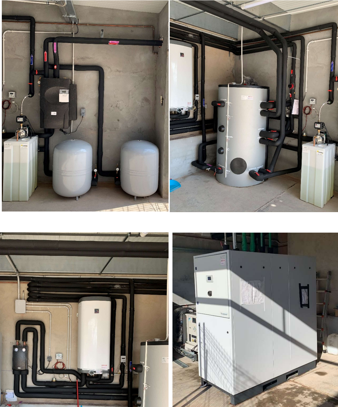
Figure 11. HYBUILD equipment room in Almatret: solar pumping station (top-left), buffer tank (top-right), DHW tank (bottom-left), and sorption chiller (bottom-right)
