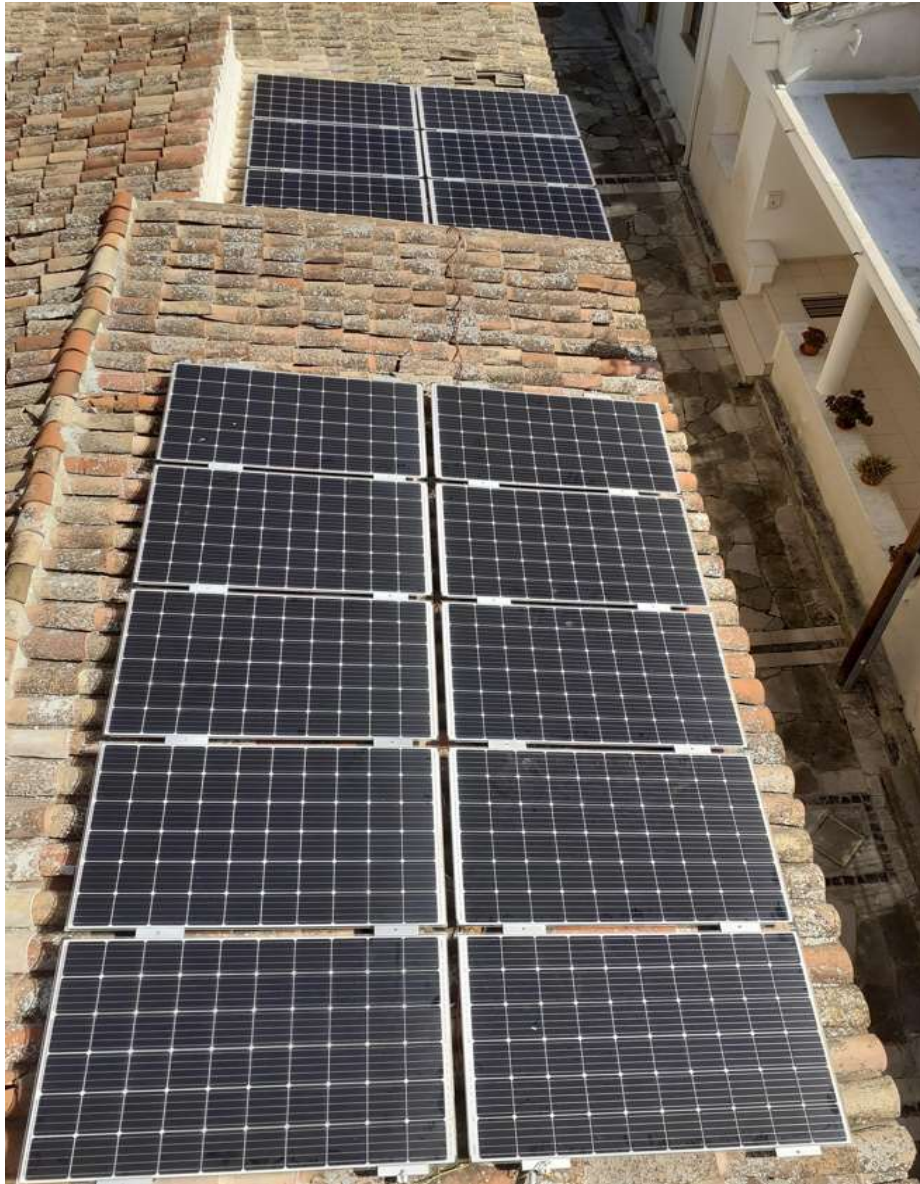
Figure 19. PV panels in Aglantzia
