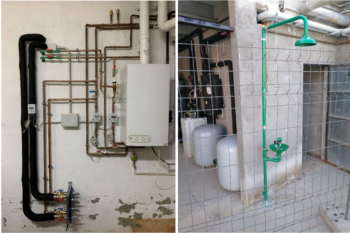
Figure 13. Connections to the gas boiler (left) and emergency shower (right) installed in Almatret
