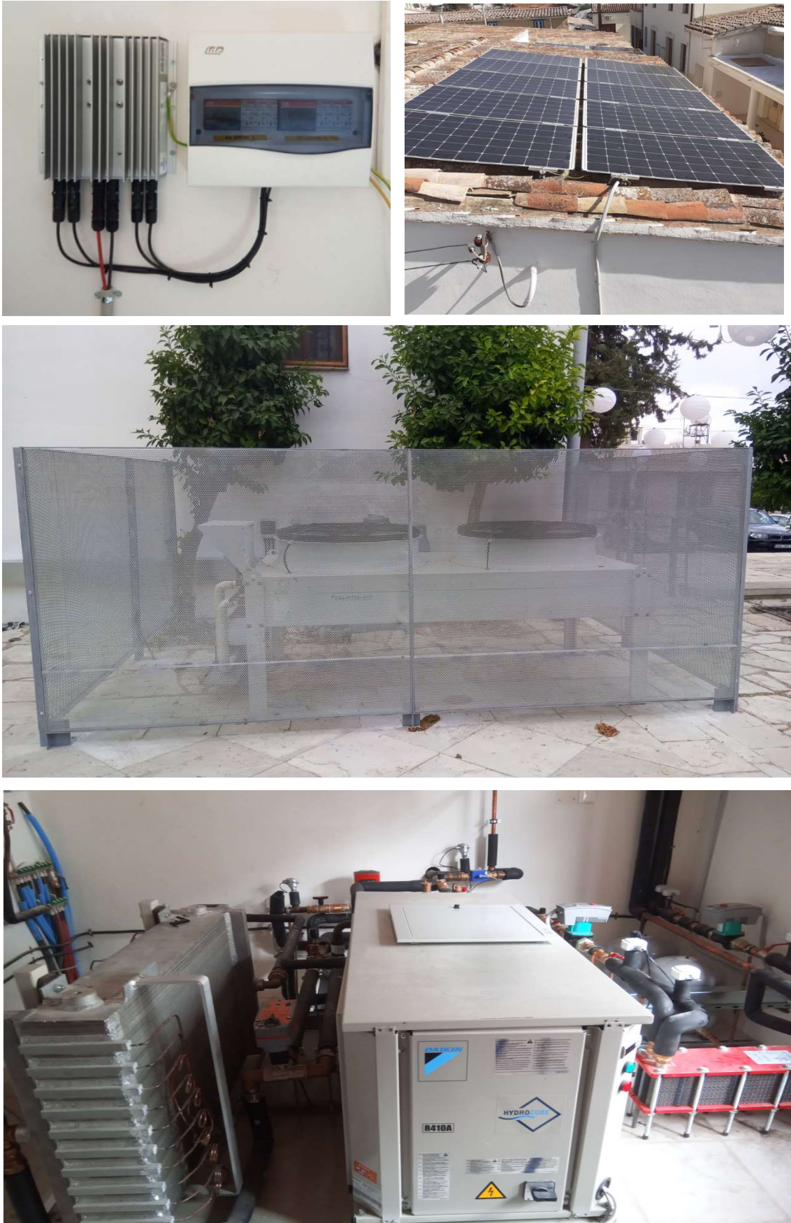
Figure 20. HYBUILD system components in Aglantzia
