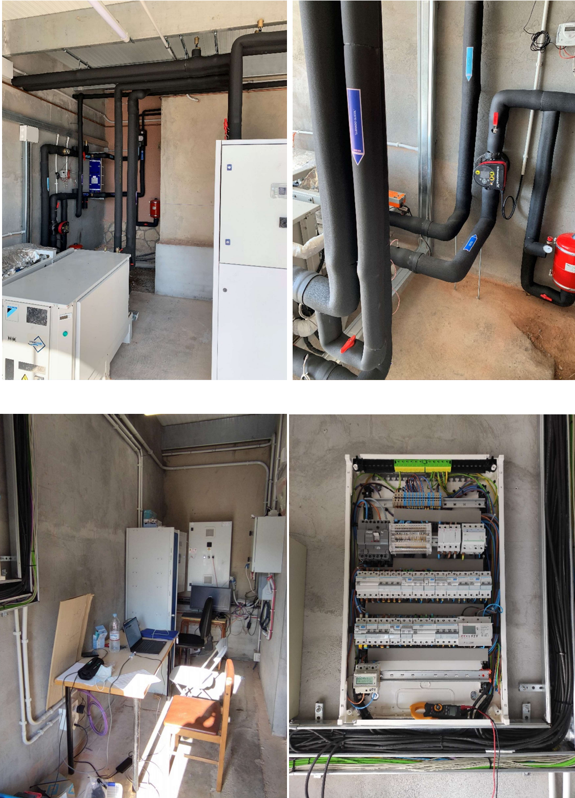
Figure 12. Equipment and control room in Almatret: heat pump hydraulic connections (top picture), control room (bottom-left), and PLC components (bottom-right)
